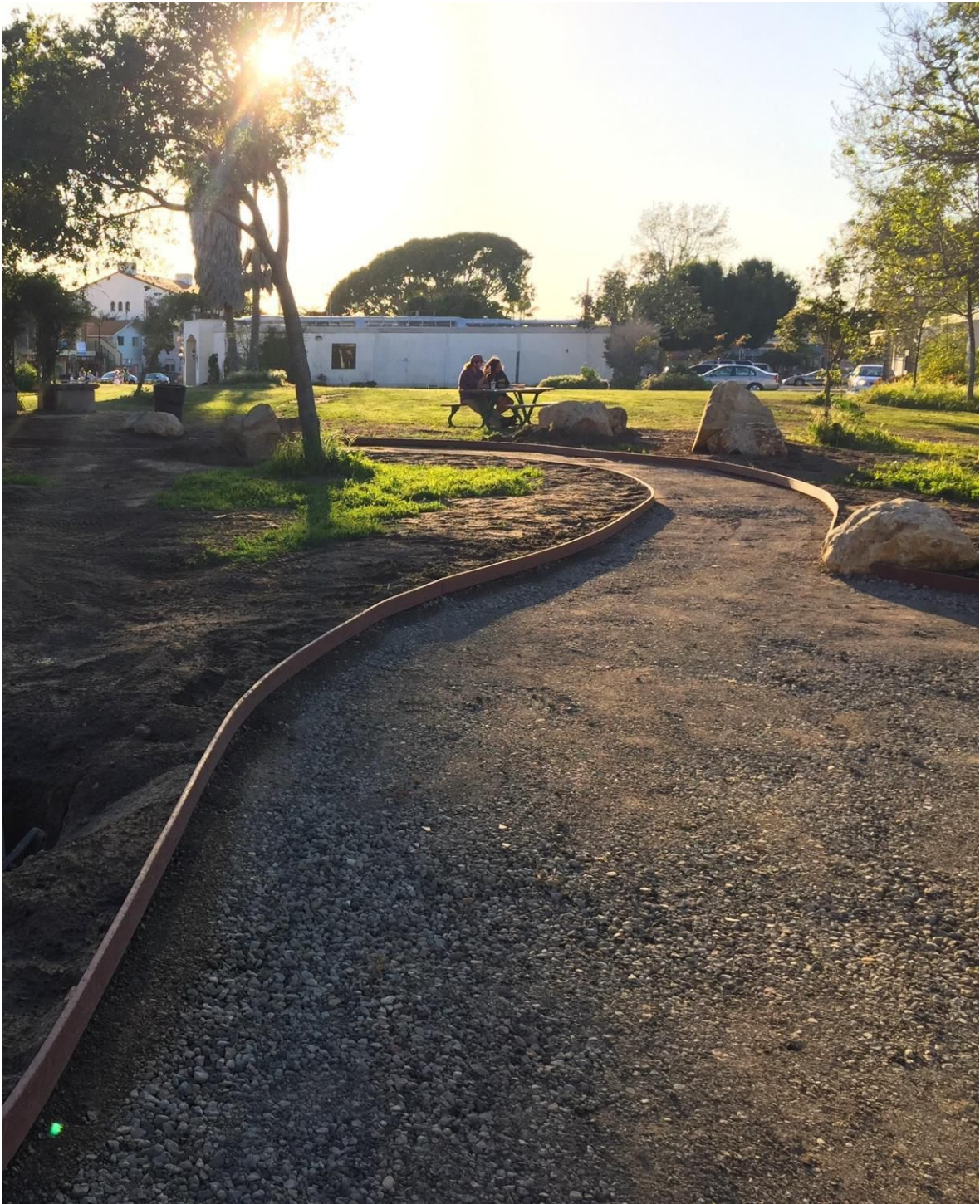
(Above) Garden pathway installation by the staff of the IV Rec and Parks District, March 2015
